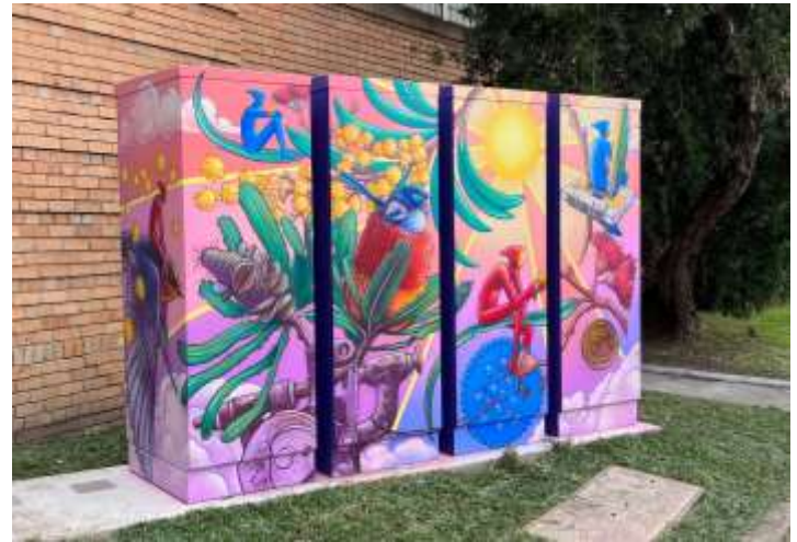
Photo of our Fitzroy North community battery , the first inner-urban community battery in Australia.
