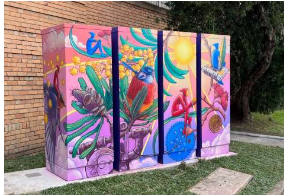
Photo of our Fitzroy North community battery , the first inner-urban community battery in Australia.
